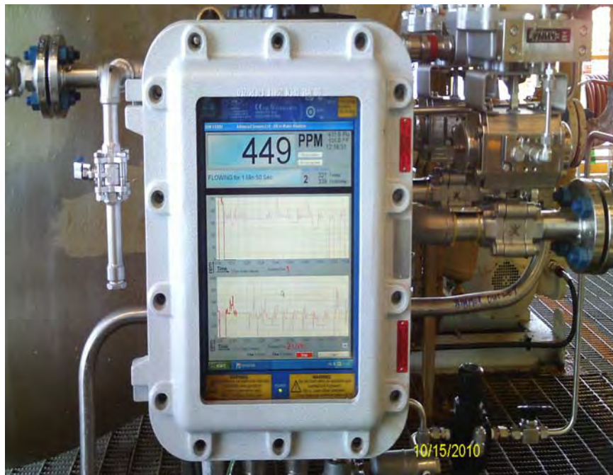
Figure 7: O&G Concentration of 449 PPM at the Skimmer Inlet.
