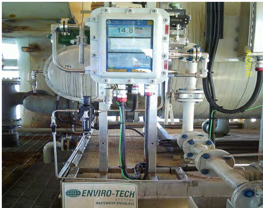
Figure 16: O&G Concentration of 14.8 PPM at the Enviro-Cell Outlet.
