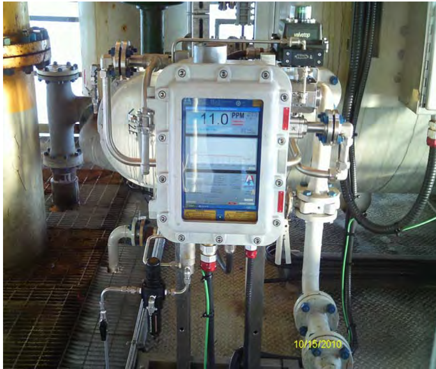
Figure 15: O&G Concentration of 11 PPM at the Enviro-Cell Outlet.
