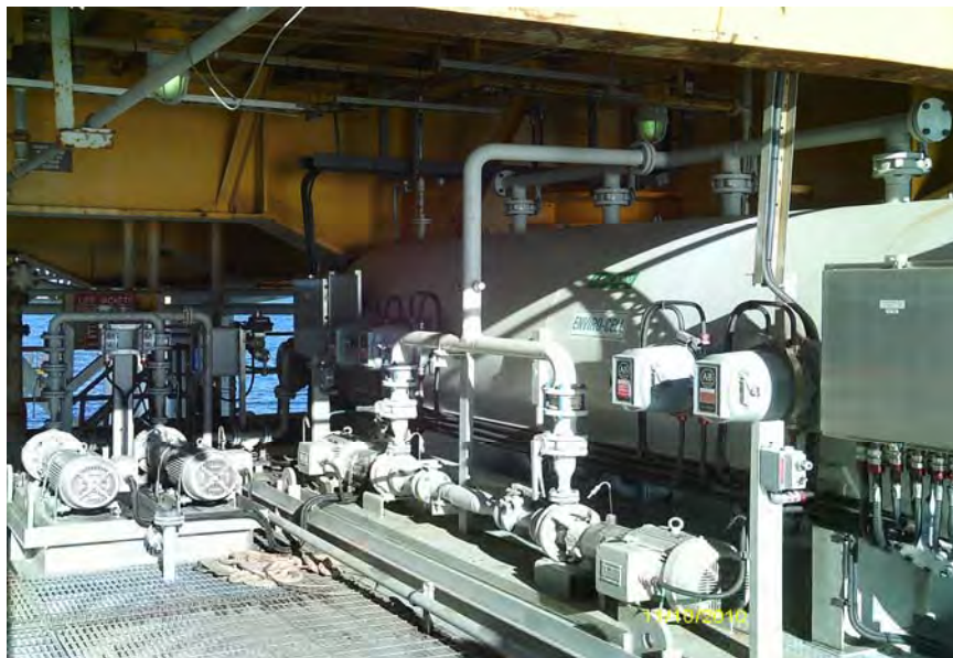
Figure 2: Enviro-Cell unit installed on the platform.
