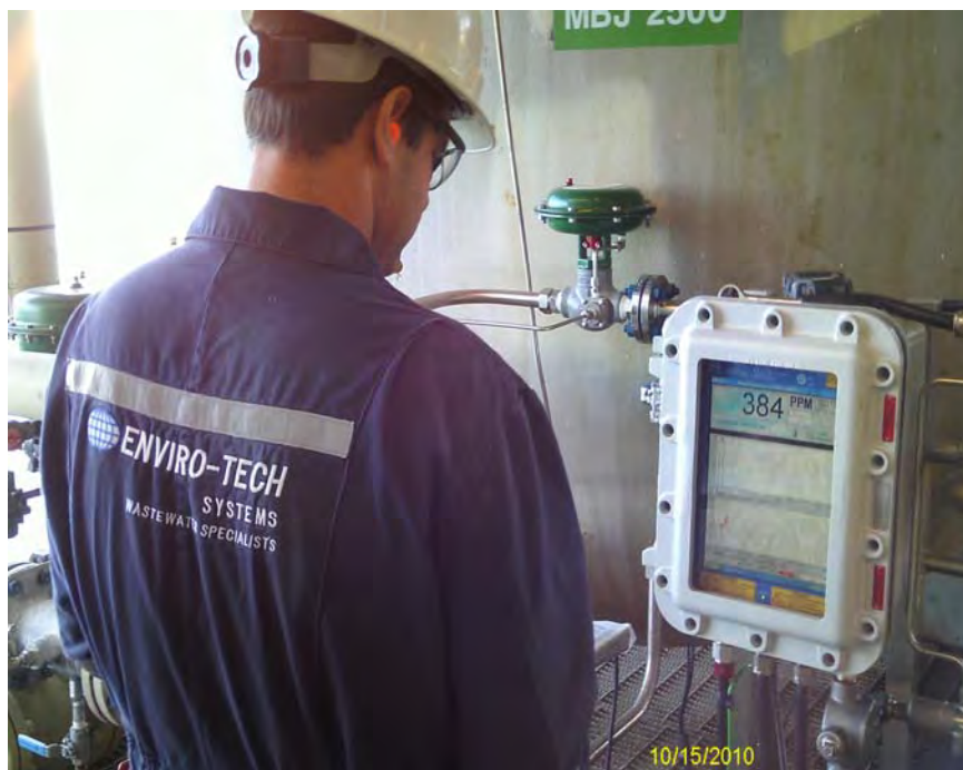
Figure 8: O&G Concentration of 384 PPM at the Skimmer Inlet.
