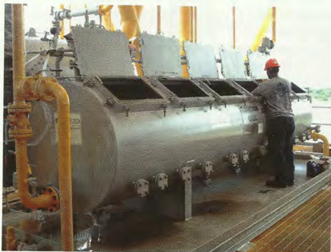
Fig. 2—An induced gas flotation unit.
